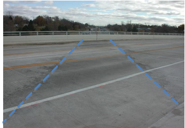
Figure 15 Bridge deck showing ECC link-slab (between dashed lines) after bridge re-opened to traffic
