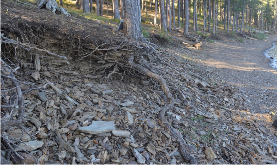
Figure 3. Bank as pictured after the 2019 erosion event. Note the talus of rock fragments from the high-water erosion event earlier that year. Talus from the 2015 high-water erosion event is to the right and has weathered into smaller fragments and gravels.
