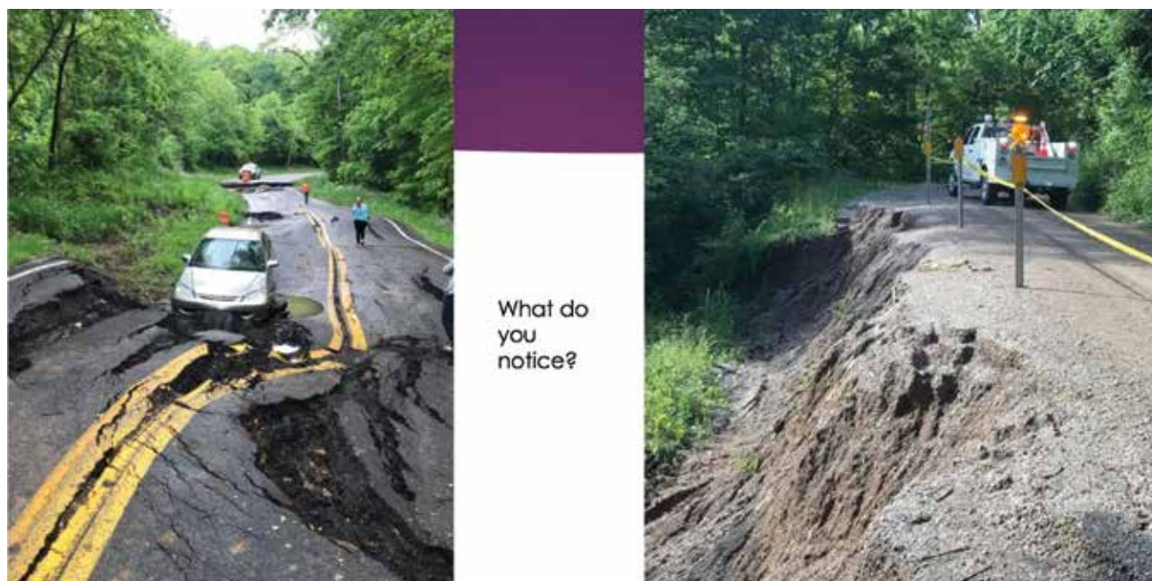
FIGURE 1: Landslide examples for introductory discussion. Left panel: vehicle stuck on a landslide-damaged portion of highway after driver drove around barricades into the closed work zone in Washington County, Ohio. Right panel: Slump caused by flooding undercutting the banks in Athens County, Ohio.
