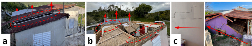
Fig. 4. Damage photos showing (a) roof envelope, (b) roof-to-wall connection, and (c) shear wall failure modes after Hurricane Maria (2017). [Photos from Emily Alfred].
