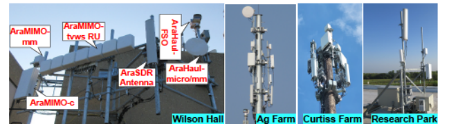
Figure 4: Physical BS installation
