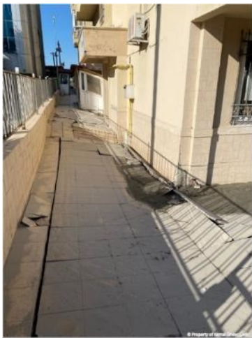
Figure 19. Ground deformation to the west of Building G (36.5904N 36.1790E; 15 FEB 2023).
