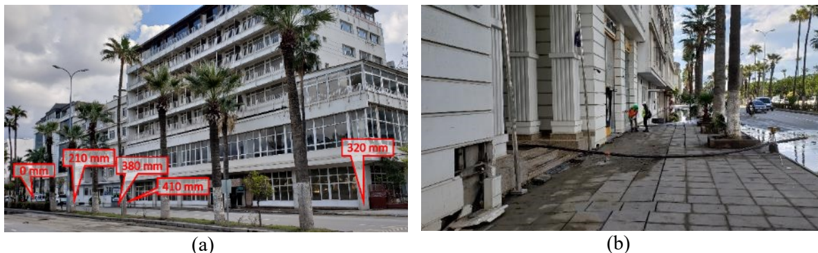
Figure 8. (a) Photo of adjacent buildings Q, R, and S with settlement measurements (36.5924N 36.1690E; 1 APR 2023), (b) same group of buildings with Building Q in the foreground and including standing flood water on front sidewalk in front of buildings R and S (36.5916N 36.1700E; 1 APR 2023).
