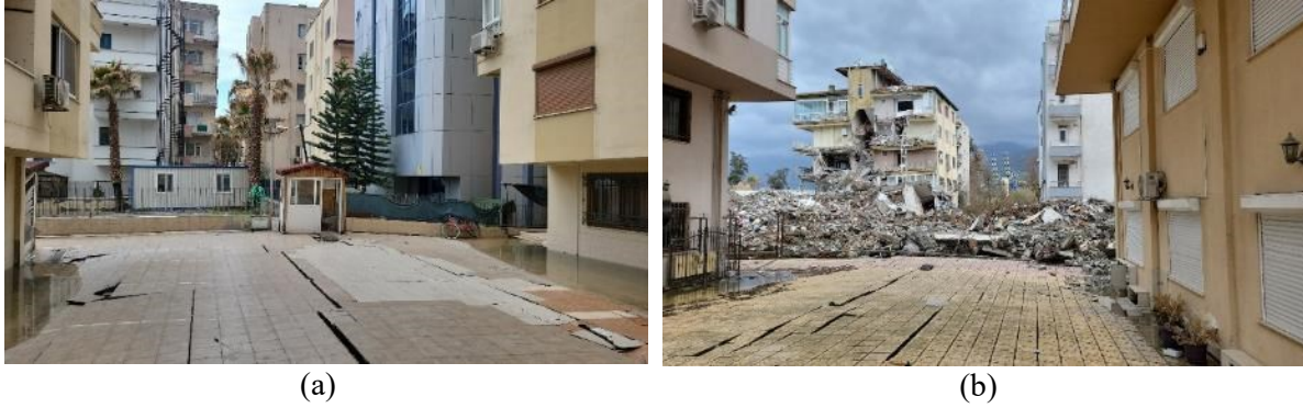
Figure 14. Building-ground interactions between four buildings in the Çay district resulting in hogging ground deformation (a) facing west with Building G on the left and Building J on the right; (b) facing east with Building I on the left and Building H on the right. Both photos were taken from the same location (36.5906N 36.1790E; 29 MAR 2023).
