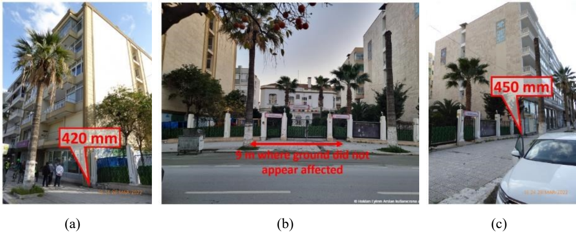
Figure 13. Buildings T, U, and V on Atatürk Boulevard in İskenderun. (a) Building to the east of Building U (Building T) where liquefaction-induced settlement caused hogging deformation to the nearby ground (36.5928N 36.1661E; 28 MAR 2023), (b) Building U, which appeared unaffected by liquefaction (36.5935N 36.1660E; 16 FEB 2023). (c) Building to the west of Building U (Building V) where liquefaction-induced settlement also caused hogging deformation to the nearby ground (36.5928N 36.1661E; 28 MAR 2023). The photo in Figure 12b is credited to Eylem Arslan and retrieved from SiteEye.
