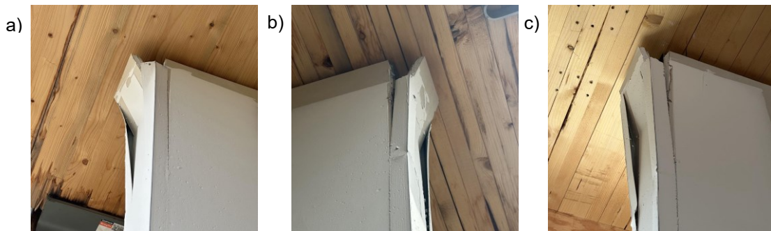
Figure 8. End of wall panel damage: (a) W6, (b) W5, (c) W16
