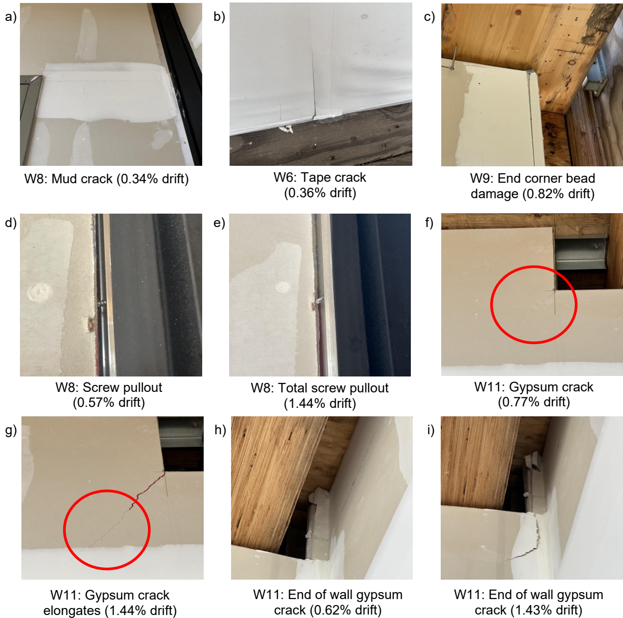
Figure 14. Observed damage to partition walls and expansion joint on Story 4 at various stages of testing.
