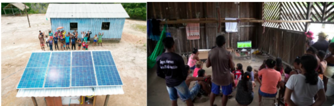
Fig. 5. Co-implementation of the solar panels at Cachoeirinha do Mentai. Left: Solar panels and other components of the technical system, with community members and research team in the background. Right: Community members and the research team use solar energy to power a TV and watch the national soccer team score the first goal of the 2022 World Cup live! (Right) (Photos: Renato Chalú, left; Wesley Braun, right).
