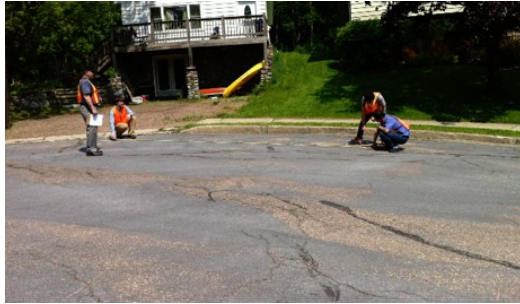
a. Orchard Terrace cul-de-sac with pavement distress indicating possible storm sewer issue
