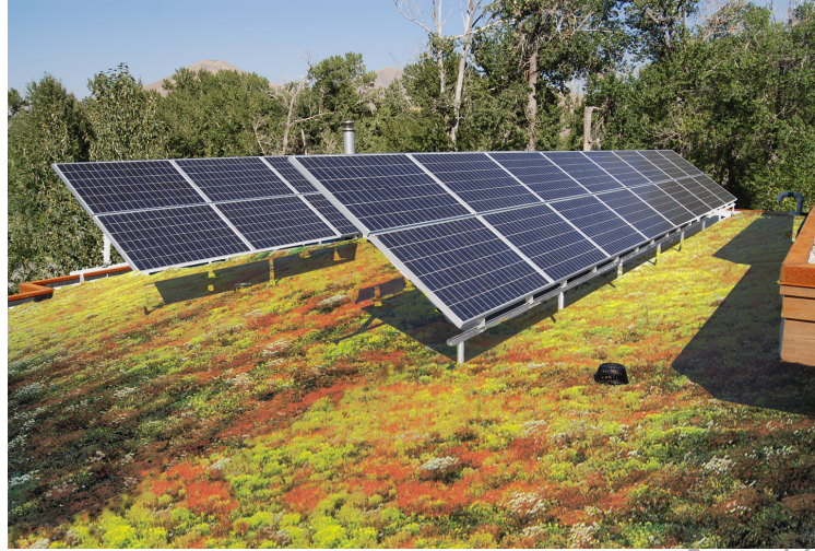
Figure 1: GR integrated PV panel installed over a rooftop in Hailey, Idaho (SVS, 2017).
