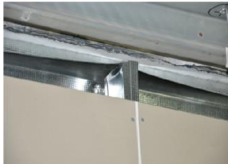
Figure 4: Lateral movement of stud from the top track on slip track partitions [14].
