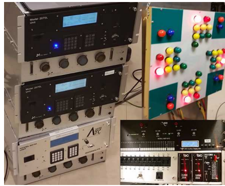
Fig. 3: Traffic Signal System in the municipality test lab. The left side shows a group of Model 2070 ATCs. The right top of the figure shows the traffic signal bulbs while the right bottom of the figure shows the CMU-212.
