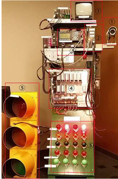
Fig. 4: Our Traffic Signal System of TS-2 Standard Equipment. The ① is a vehicle detection and surveillance system. The ② shows the MMU-16LE while the ③ shows the Siemens Model 60 ATC. The ④ and ⑤ indicate the Load Switch relays and traffic signal bulbs, respectively.
