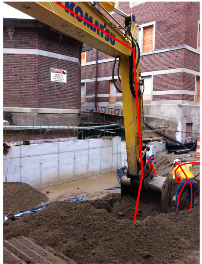
Fig. 1. Illustration of the 2D on-site pose estimation system on a video frame for both articulated construction robot and human workers. Red lines are the estimated pose. (For interpretation of the references to colour in this figure legend, the reader is referred to the web version of this article.)
