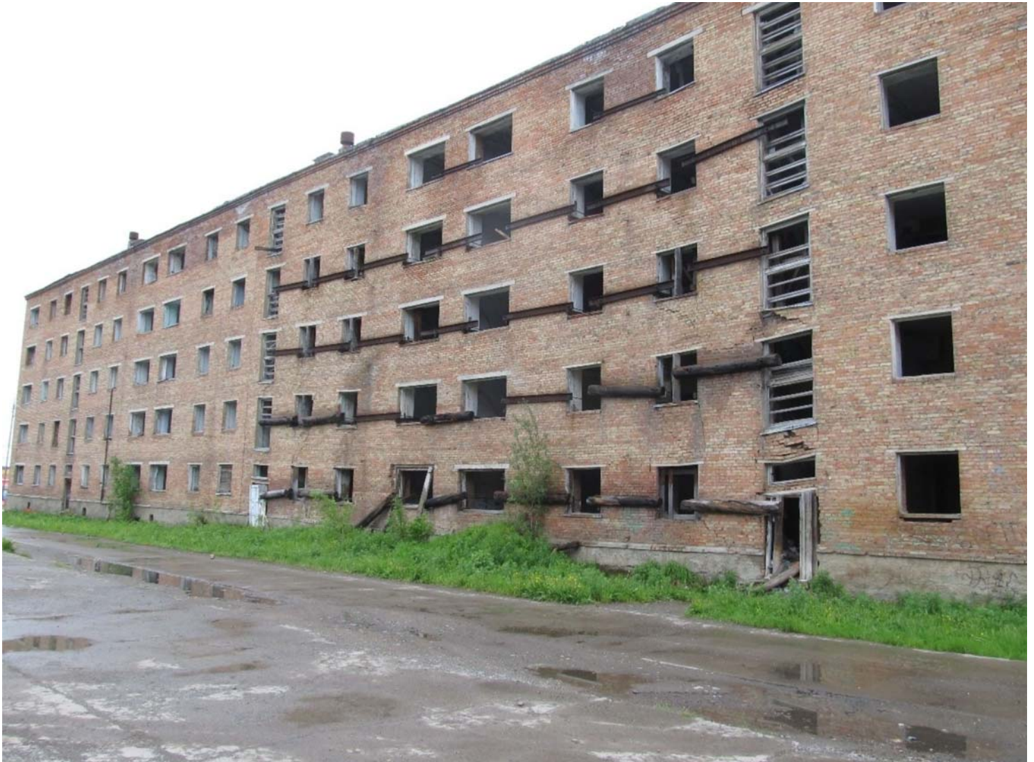
Figure 3. Example a block-style building in Igarka suffering from severe structural instability caused by thawing permafrost (Photograph by: Dmitry Streletskiy, 2011).
