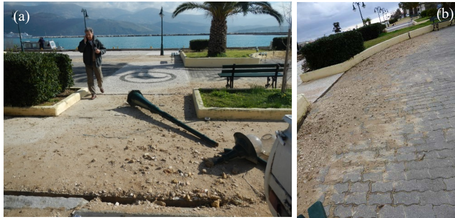
Figure 1: Examples of gravelly soil liquefaction through pavement construction joint at the port of Lixouri following the second earthquake. Note the large particle size of the ejecta (a): 38^{\circ}11'55.38''\text{N} , 20^{\circ}26'20.98''\text{E} ; (b): 38.199166 , 20.439166 .
