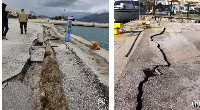
Figure 3: (a) Displacement of the quay wall in Lixouri port, across the Plaza of National Resistance following the second earthquake (GPS coordinates: 38.199444, 20.439444); (b) displacement ( \sim 16 cm) of the quay wall in Argostoli port.
