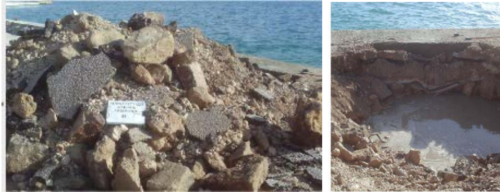
Figure 4: Views of debris excavated adjacent to the port seafront at the location where the maximum lateral displacement of the quay walls was registered in Lixouri. The large particles of the fill material is visible. (Geoconsult Ltd, 2016)
