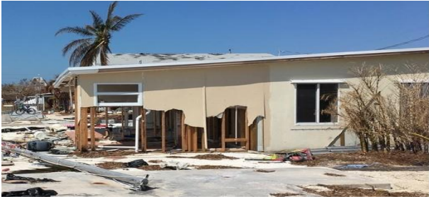
Figure 6a: surge damage to walls
