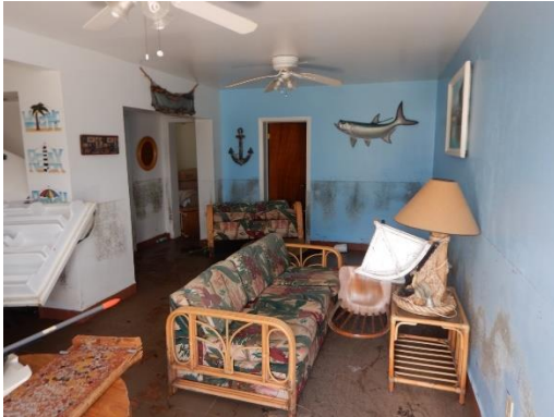
Figure 1a: Interior Damage
