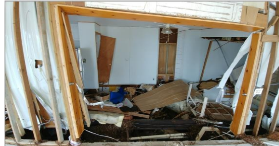
Figure 6b: surge interior damage
