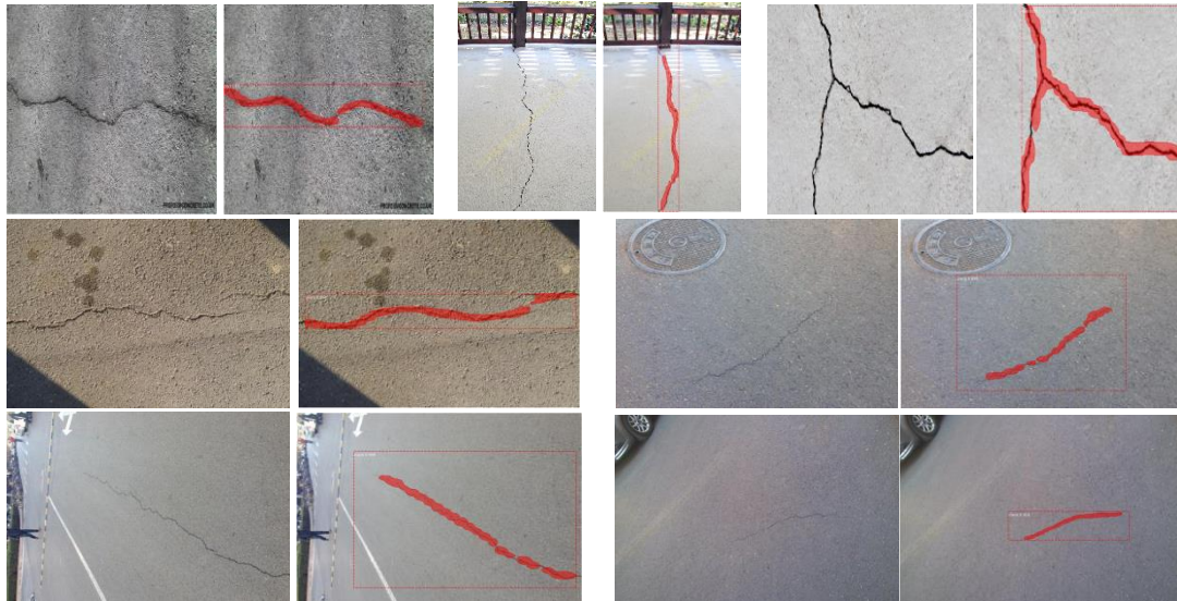
Figure 6. Examples of crack detection on test images
