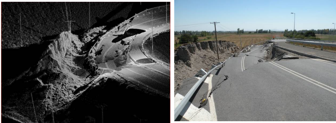
Figure 2. Ground-based LIDAR and optical images of a failed overpass embankment on Ruta 5 from the 2010 Chile Earthquake (LIDAR survey by Kayen presented in Bray and Frost 2010).
