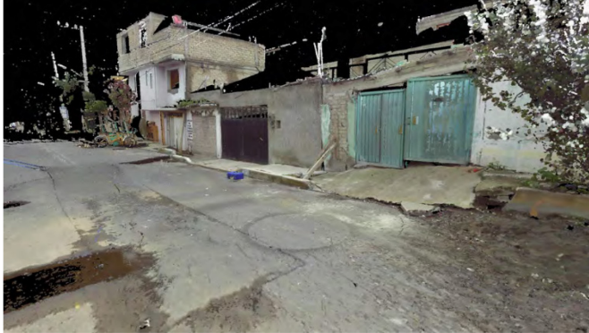
Figure 8. LIDAR model showing ground failure in Colonia del Mar (N19.2851°, W99.0579°; Mayoral et al. 2018).
