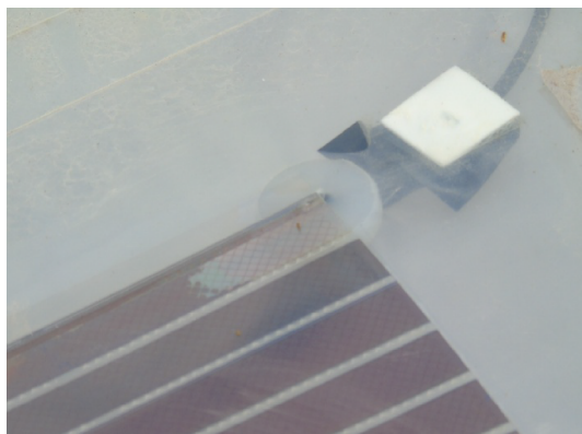
Fig. 13. Degradation at the cable connection of the OPV panel.
