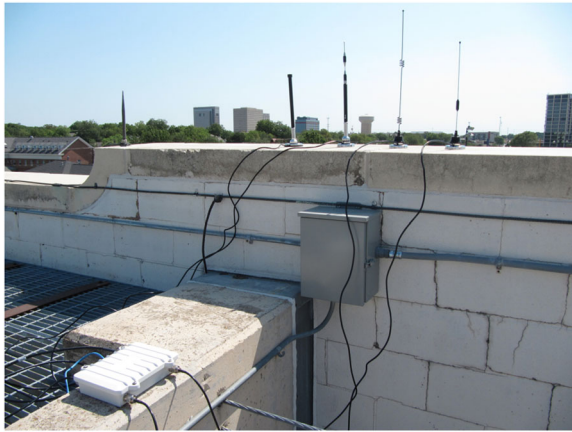
Fig. 9 Gateworks board with four Ubiquiti radios and antennas at 900 MHz, 2.4 GHz, and 5.8 GHz on top of a parking garage on campus. This figure shows the in-field experiment set-up
