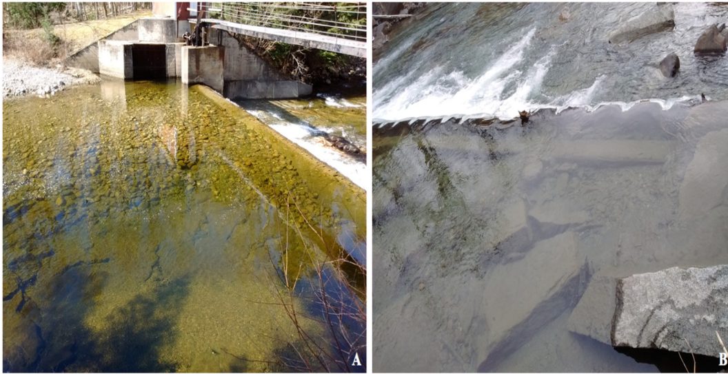
Fig. 7. (A) Reservoir at WAM. Half of the reservoir behind the dam is dominated by a scour pool over 1 m deep. The other half is dominated by a coarse-bedded sediment ramp that slopes up to the dam. (B) Reservoir just behind the dam at SOR. Sediment is built up on average approximately 40 cm below the dam crest for 100 m behind the dam. (Color figure available online)
