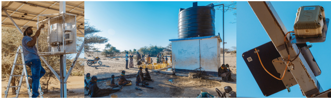
Fig. 1. A typical groundwater borehole in Turkana, Kenya (center). Electrical monitoring sensors are installed at the pump controller (left), and wireless transmit data to a self-powered satellite or cellular transmitter ( www.sweetsensors.com ).
