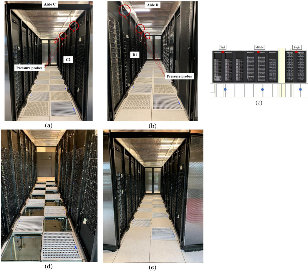
Fig. 4. (a) & (b) Experimental setup for scenarios I and II, dampers were installed in staggered layout inside aisles C and D. (c) Location of pressure sensors inside aisles C and D as well as inside the plenum at the middle of pedestals. (d) Perforated tiles were removed in aisles C and D. (e) Experimental setup for scenario III, new layout of ES2 data center with solid tiles.
