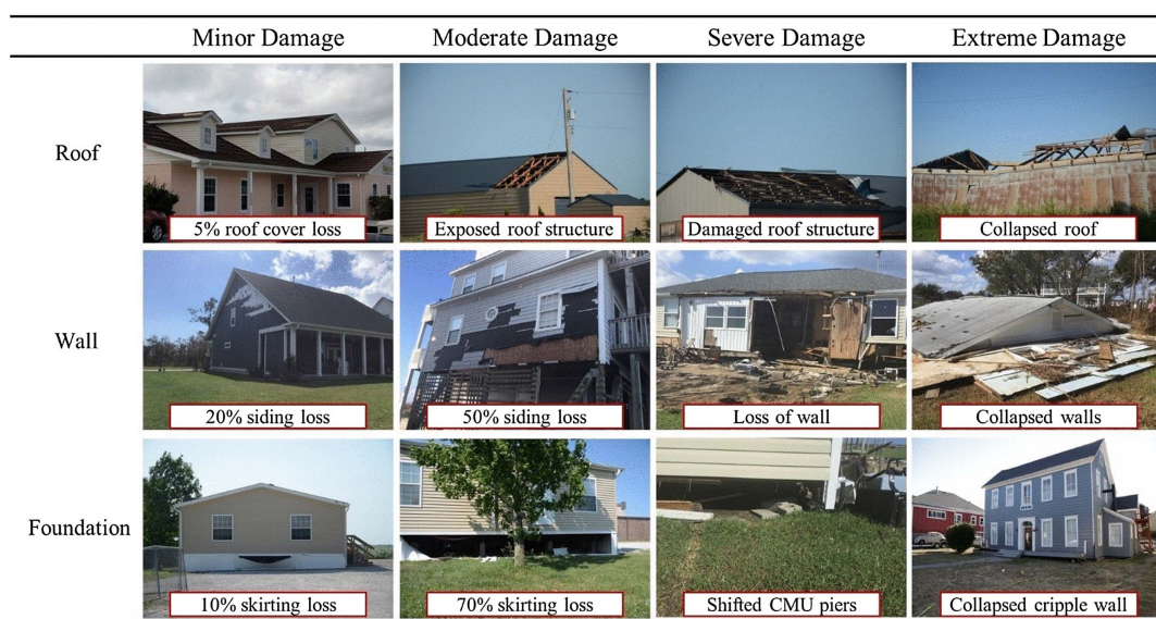
Fig. 3. Classifications for structural damage, except nonbuilding structures (e.g., grain bin) which were classified as extreme damage if any damage was apparent. (Images by authors.)
