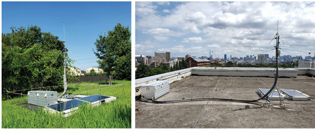
Fig. 3. Typical LMA installations on the ground (left panel: Kumagaya Station) and roof-top (right panel: Toyama Station). The stations are solar powered and operate on a fully stand-alone basis, communicating their data via cellular data modems to a central processing server. The rectangular enclosure houses deep-cycle batteries and a sealed electronics box containing the VHF receiver, data processor, GPS, cellular data modem, and solid-state disk. The stations were specially designed by NIED to be rugged and low-profile to withstand typhoons.
