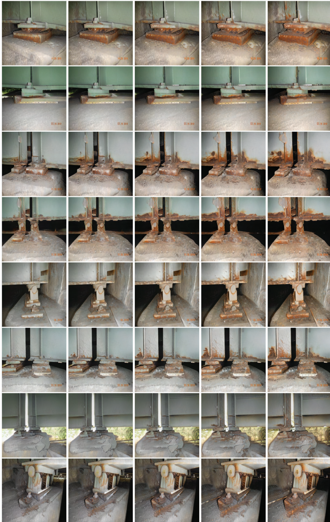
Figure 17. Examples of synthetically generated images with semantic corrosion forecasting
