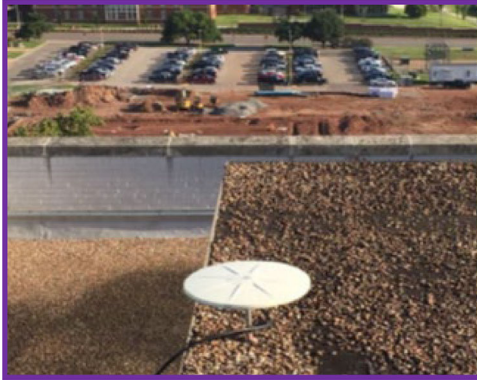
Figure 5. GPS antenna mounted on the roof.
