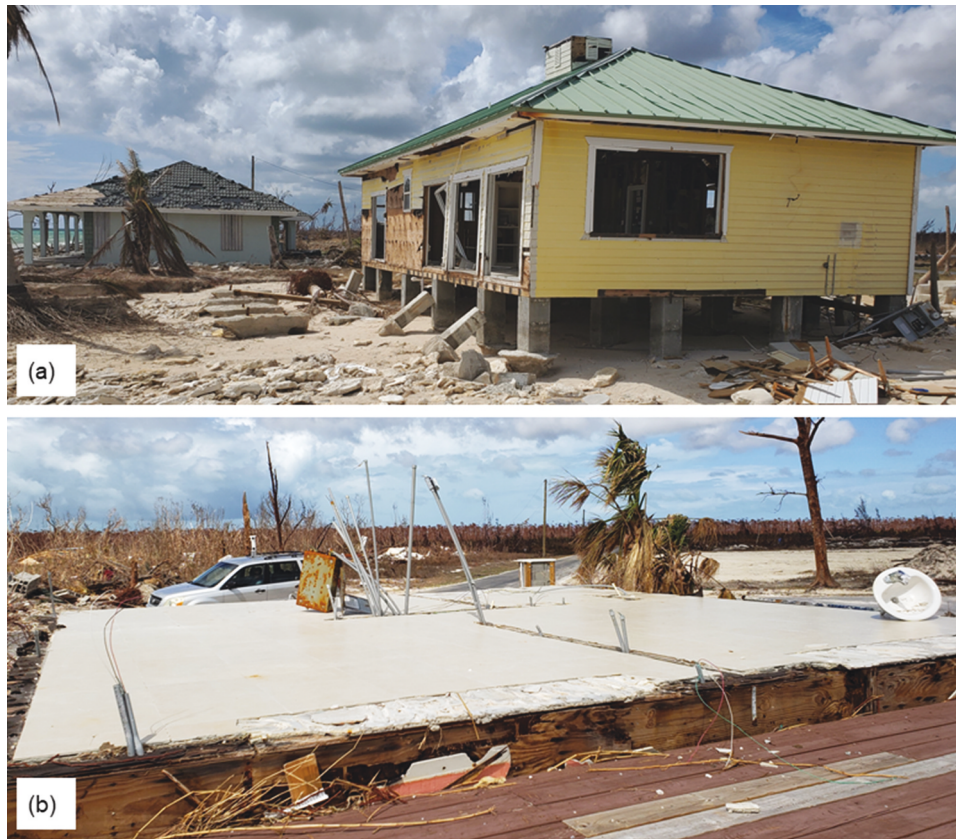
Figure 15. Examples of varying damage levels observed in Class 2 wood-framed homes on elevated CMU piers in Pelican Point (Grand Bahama Island), including (a) surge wash-through of a single-story wood-frame home at (26.649183, -78.092826); note that a deck present on the coast-side of the home was removed but could not be found in nearby debris piles; and (b) complete destruction of the superstructure of a wood-frame home built atop a wood floor platform supported by CMU piers (26.649183, -78.092826).
