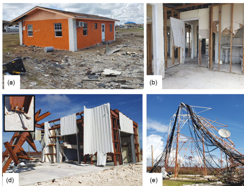
Figure 14. McLean's Town Cay (Grand Bahama Island) overview: (a) surviving Class 2 structure at (26.648639, -77.947904) with good wind resistance but (b) extensive interior damage due to storm surge; Examples of failures in other structural classes: (c) steel marine facility at (26.646725, -77.952984) with inset of anchor failure and (d) lattice communication tower at (26.648297, -77.947030).
