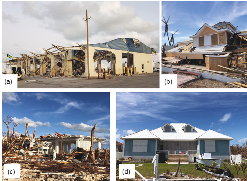
Figure 11. Illustrative performances in the Marsh Harbour (Great Abaco Island) region: (a) failure of masonry infill on steel moment frame port warehouse at (26.542944, -77.064664); (b) example of surge-induced “soft story” failure in wood framed Class 2 residence at (26.545954, -77.046597); (c) complete destruction under storm surge leaving only the elevated foundation of an assumed Class 3 home at (26.551910, -77.037554); and (d) minor/no structural damage in a coastal Class 3 masonry home at (26.552433, -77.060514).
