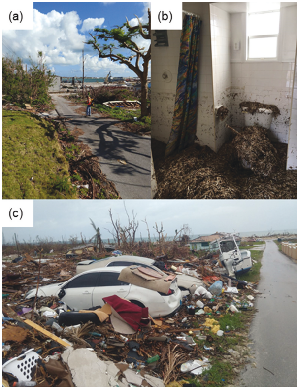
Figure 3. Representative high water marks. (a) Looking downward from approximately 8.1 m HWM in Marsh Harbour, Great Abaco; (b) Interior watermark in bathroom; (c) Looking seaward from 6.2 m elevation near top of large debris pile/watermark on the side of a hill in Marsh Harbour.
