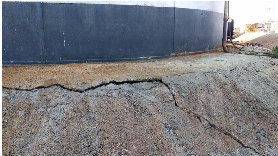
Figure 6. Cracking of the concrete blind area of the tank. Photograph by F D Yurov. Reproduced with permission.
