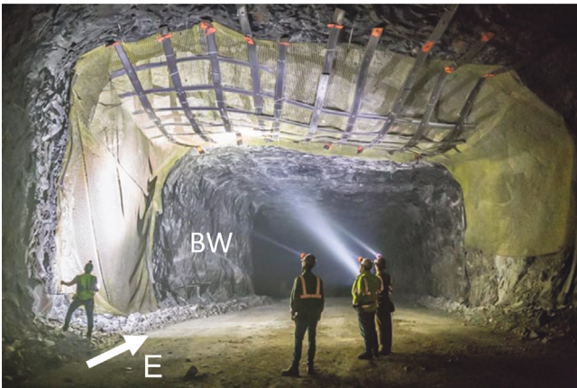
Figure 2. Mitigated large cave in the southern tunnel of Figure 1. The tunnel wall on the left of the photo is the south wall (BW) of the pillar. From Baggett et al. (2020).
