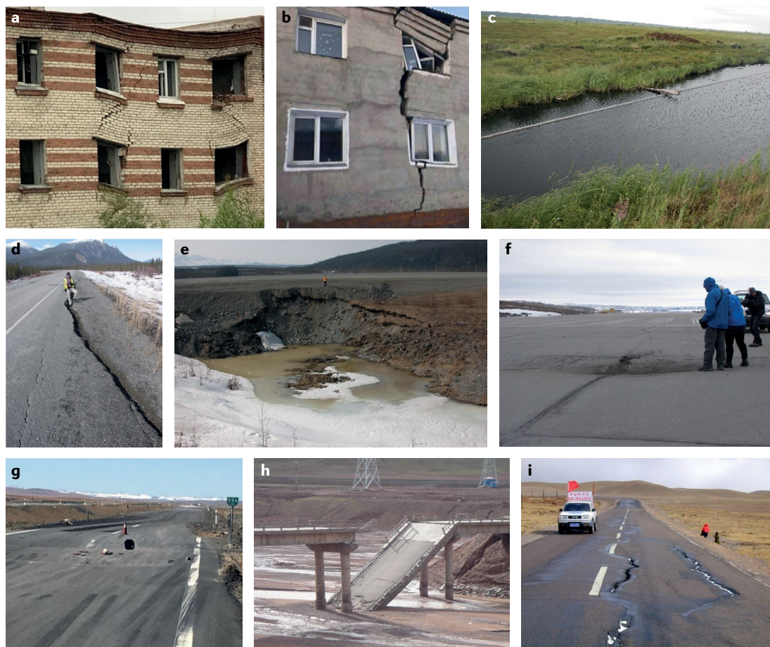
Fig. 3 | Infrastructure damage owing to degradation of permafrost. a–c | Infrastructure damage in Russia, including damaged buildings in Yakutia (panels a and b ) and a below-ground pipeline crossing an area with ice-rich permafrost and thermokarst development in Yamal-Nenets (panel c ). d–f | Infrastructure damage in North America, including longitudinal cracking due to shoulder rotation along the Alaska Highway in Yukon, Canada (panel d ), thermokarst affecting the embankment of the Alaska Highway in Yukon, Canada (panel e ) and a sinkhole in the Iqaluit runway (Nunavut, Canada) (panel f ). g–i | Infrastructure damage in the Qinghai-Tibet Plateau, including embankment deformation of Gong-Yu Express Highway (panel g ), a collapsed bridge of Qinghai-Tibet Highway (QTH) (panel h ) and longitudinal cracks of QTH (panel i ). Panels a and b courtesy of Ivan Khristoforov, panel e courtesy of Eva Stephani and panel g courtesy of Chen Ji.
