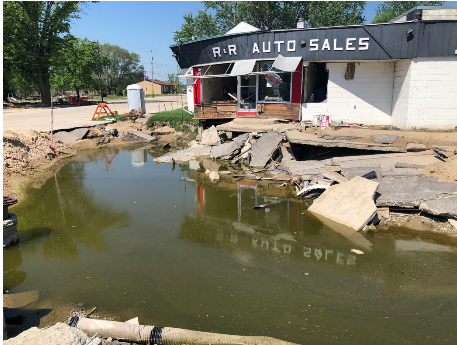
Figure 5: Sidewalk and road failure plus foundation damage due to scour
