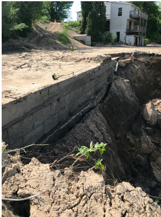
Figure 4: Exposed foundation of home near the bank of the Tittabawassee
