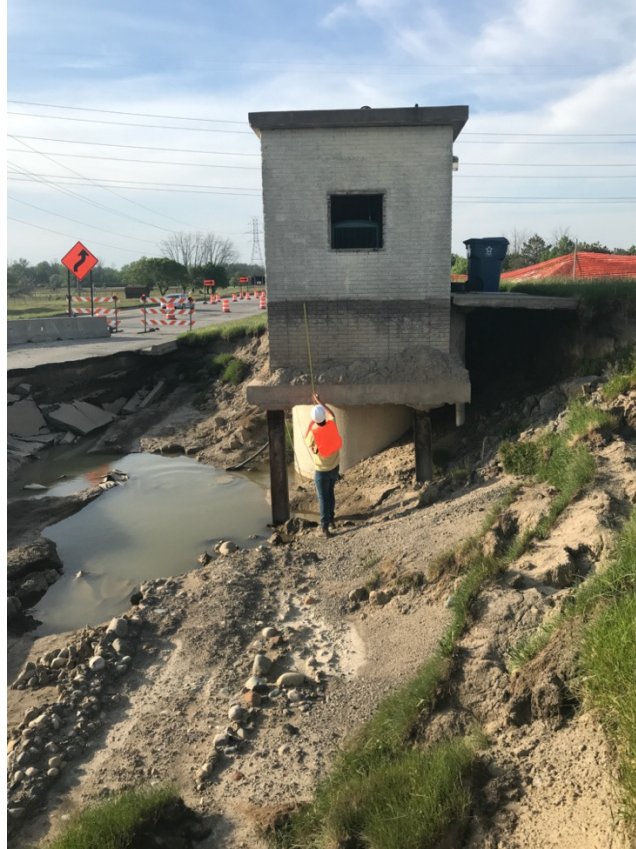
Figure 6: Poseyville Dike failure
