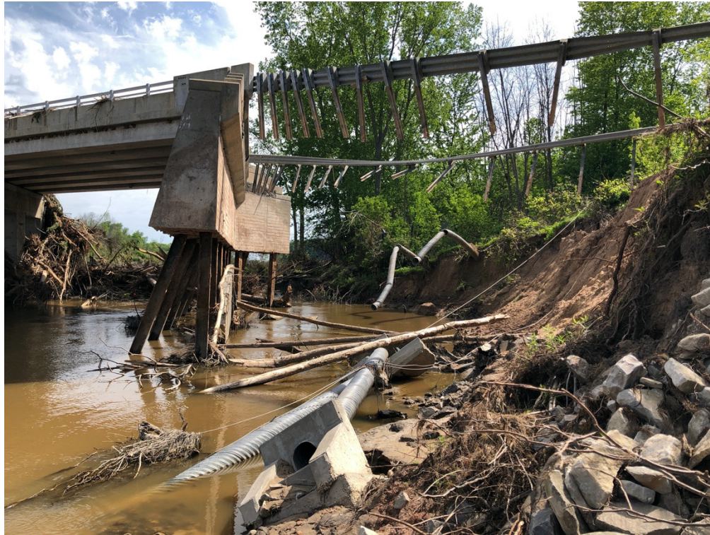
Figure 2: M-30 Bridge embankment failure
