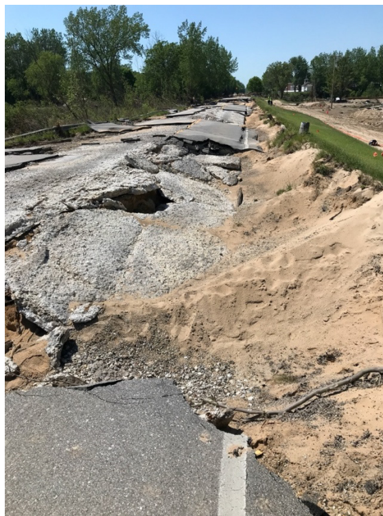
Figure 3: W Saginaw Rd approach embankment failure
