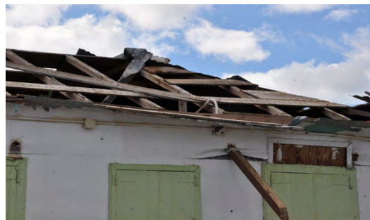
Figure 1. Illustration of roof panel loss in Puerto Rico due to Hurricane Maria (Source: FEMA, 2018a)
