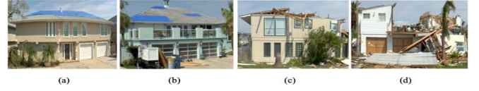
Fig. 13. (a) and (b) show buildings with temporal roof tarp and (c) and (d) show buildings with a destroyed roof.
