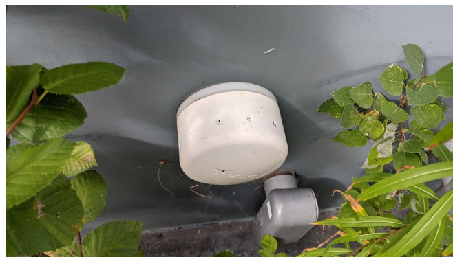
Figure A1. Detailed image of the diffuser port at station I23K in Minto Alaska. This configuration is typical of Alaska Transportable Array stations. The color version of this figure is available only in the electronic edition.
