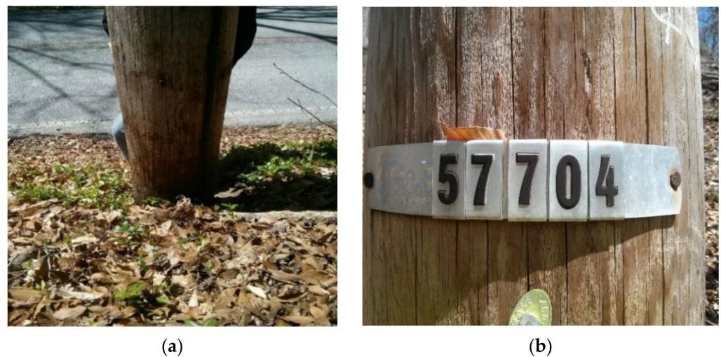
Figure 5. Tested wooden utility pole labeled as 57704: (a) its embedment condition and (b) its label.
