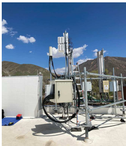
(b) RENEW hardware deployed at a new rooftop location.
