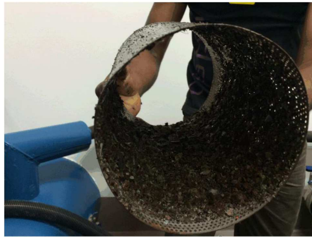
Fig. 8. Debris in the water pipe blocks the water flow, reduces the heat exchange rate drops and causes the drift of system internal irreversibility states.
