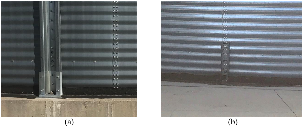
Figure 4. (a) Vertical stiffener and anchorage for Bin 5 (commercial bin). (b) Typical anchorage clip for Bins 1 – 4 (farm bins).
