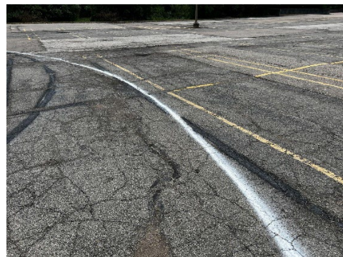
Fig. 8. Example of Poor Course Condition. Potholes and parking lot lines contributed to unwanted noise.
