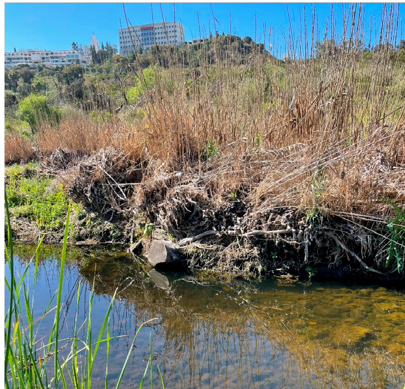
Figure 5. Bank failure within the upstream reach of Del Cerro, Alvarado Creek.
