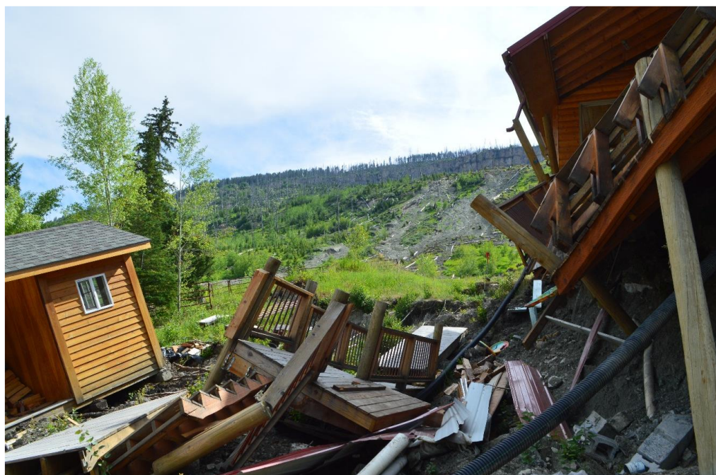
Figure 7. The mudslide occurred in one of the non-recovery areas, resulting in damage to multiple houses.
