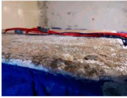
Figure 20. Final slab condition with ice formation on slab surface after misting.
