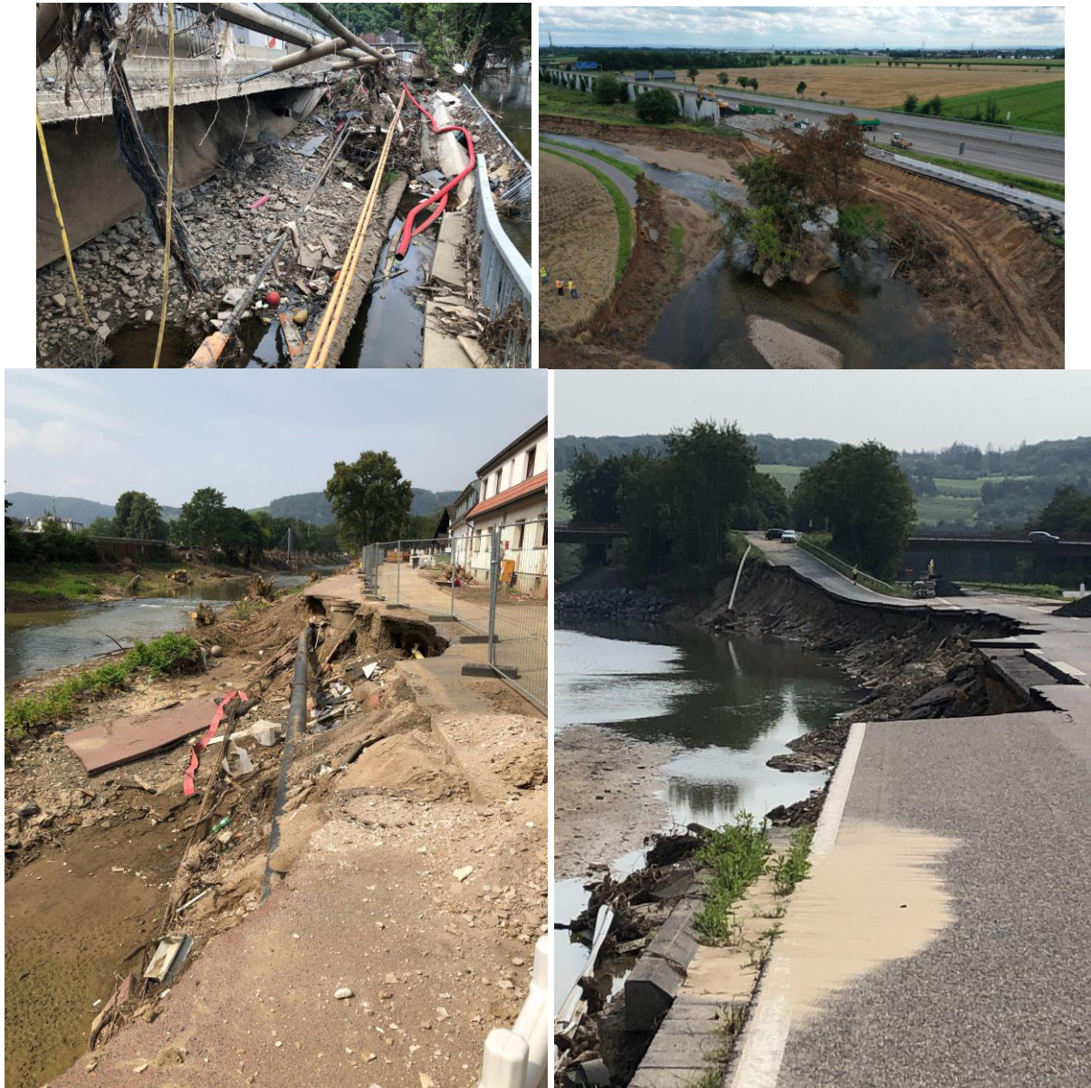
Figures 1 a-d: Observed building damage in various locations. a (Top Left): Chaudfontaine, Belgium (Lat: 50.58694, Lon: 5.65004); b (Top Right): Autobahn A1, Erftstadt-Blessem, Germany (Lat: 50.81338, Lon: 6.78907 ); c (Bottom Left): Ahrweiler, Germany (Lat: 50.53880, Lon: 7.10424); d (Bottom Right): Bad-Neuenahr Ahrweiler (Lat: 50.54669, Lon: 7.17881).
