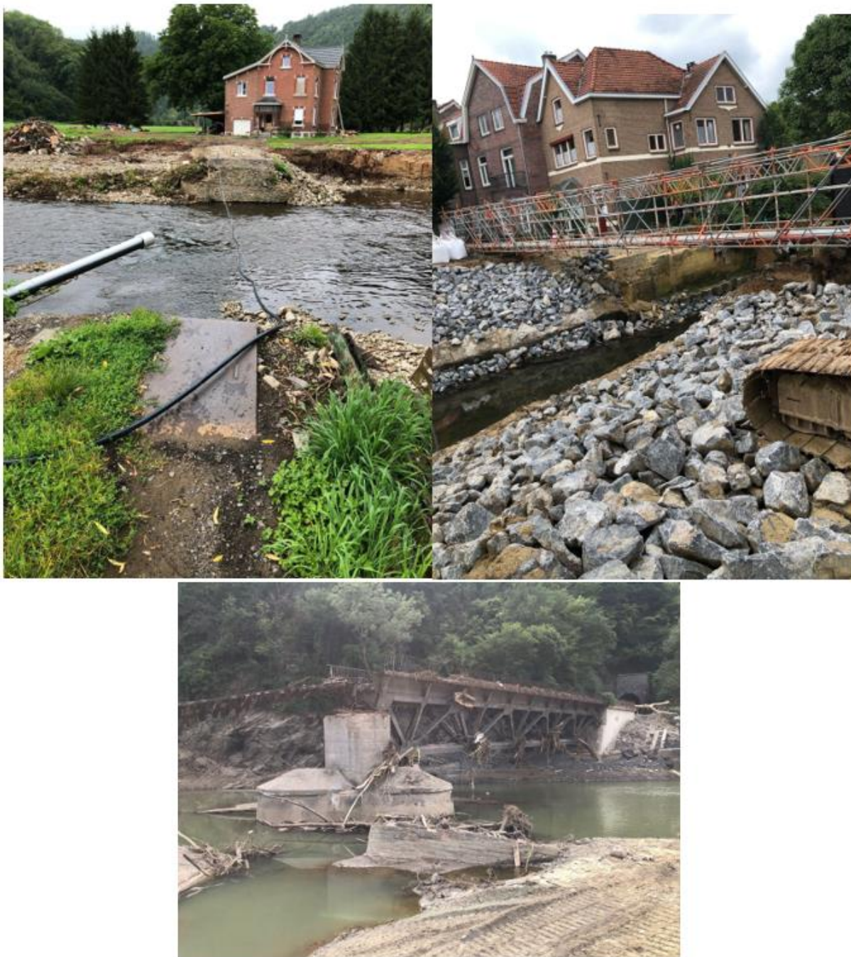
Figures 3 a-c: Three observed bridge failures observed in the reconnaissance mission. a (Top Left): Goffontaine, Belgium (Lat: 50.57217, Lon: 5.76563); b (Top Right): Valkenburg, Netherlands (Lat: 50.86523, Lon: 5.82950); c (Bottom): Mayschoß, Germany (Lat: 50.51815, Lon: 7.02690).
