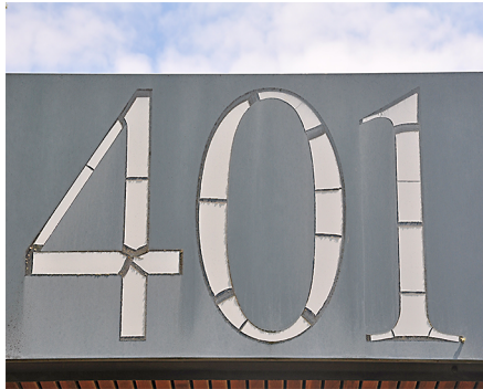
FIG. 2. Cracked lettering at Ecole Polytechnique, Palaiseau, France
