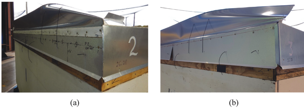
Fig. 20. Fascia lifting at a wind speed of 60 m/s (a) Configuration 2, and (b) Configuration 3.
