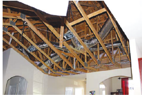
(b) Ceiling collapse due to water ingress
