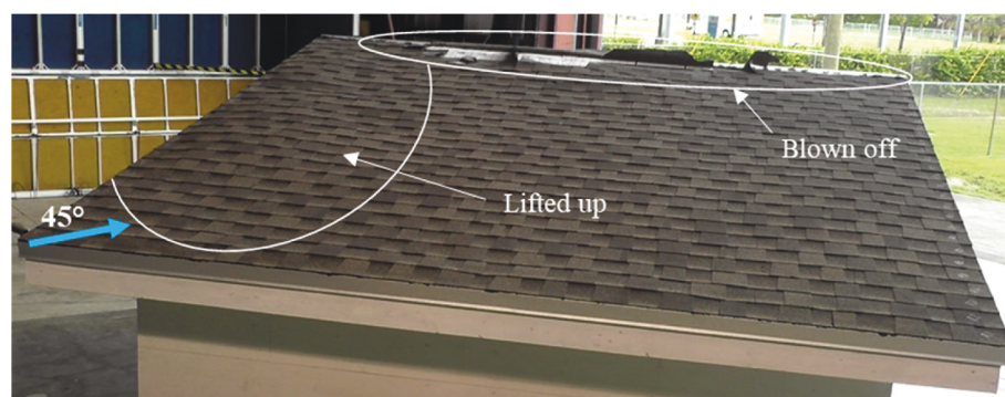
Fig. 21. Case 6: shingle blowoff at a 3-s peak wind speed of 56.8 m/s.
