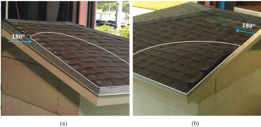
Fig. 19. Gable-end shingle failure mechanism for hip-gable roof Control 2b (a) shingle billowing in the interior parts of the roof, and (b) gable end shingle liftoff initiation.
