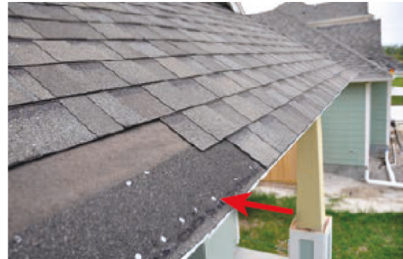
(b) Eave shingle damage
