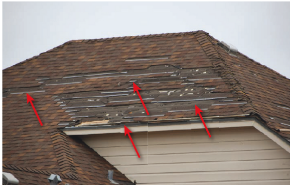
(a) Ridge-cap and eave shingle damage
