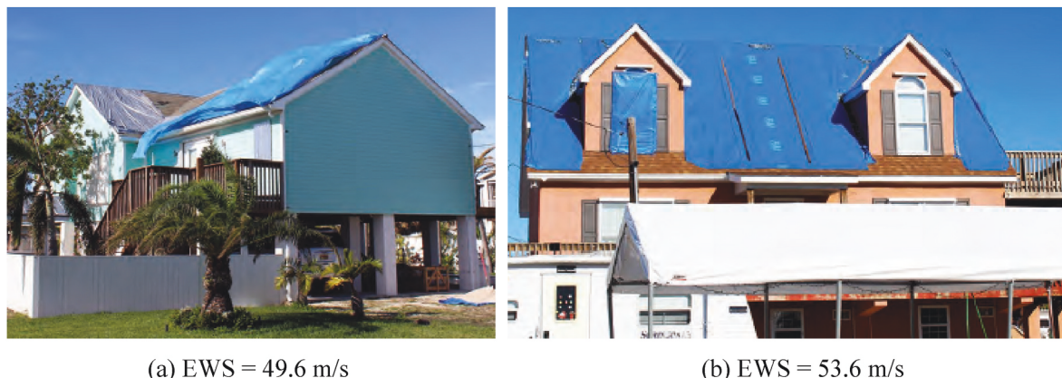
Fig. 1. Shingle damage during hurricane Irma (Source: FEMA, 2018).
