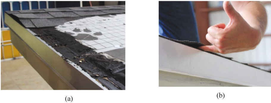
Fig. 18. (a) Gap left at the rake edge; (b) Gap between shingle layers in the headlap.
