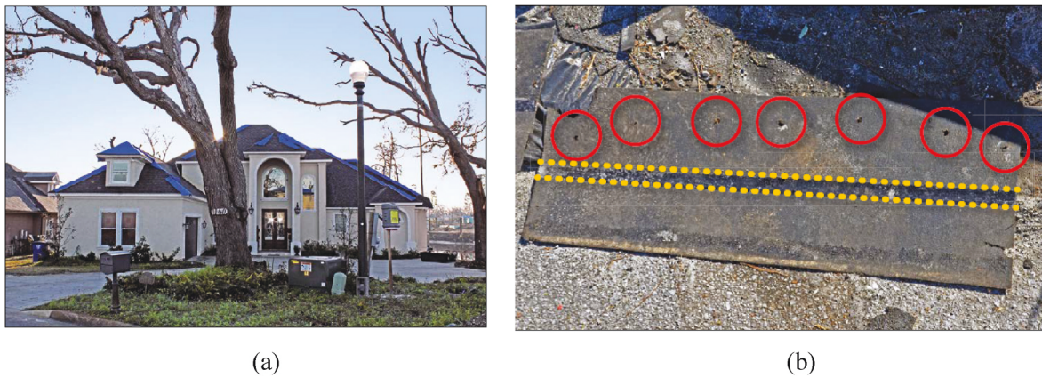
Fig. 5. Observed installation deficiencies after Hurricane Michael (a) unsealed shingles; (b) high-nailing (Source: FEMA, 2020).
