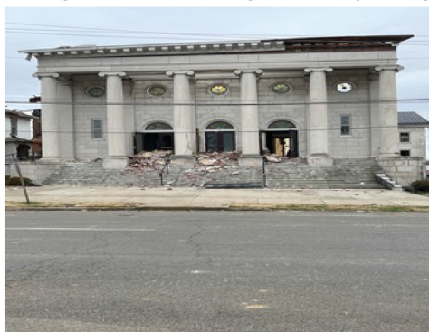
(g) Damage to the Methodist church: Destroyed
