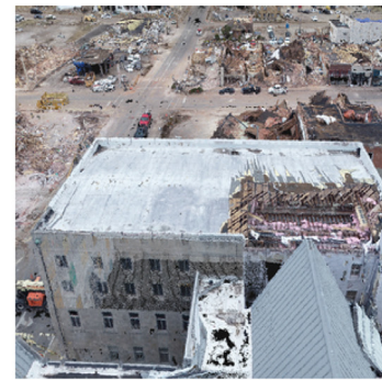
(c) Minor damages to the roof
