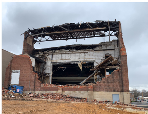
(e) Damage to the American Legion: Severely Damaged
