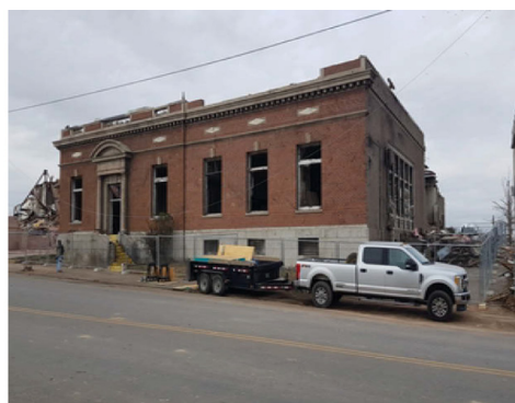
(b) US Post Office: Moderately Damaged
