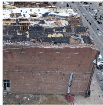
(b) Loss of sheathing
