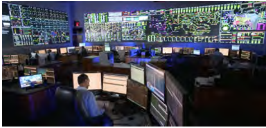
Fig. 2: Pennsylvania-New Jersey-Maryland (PJM) Interconnection control room, using numerous small multiples [17].
