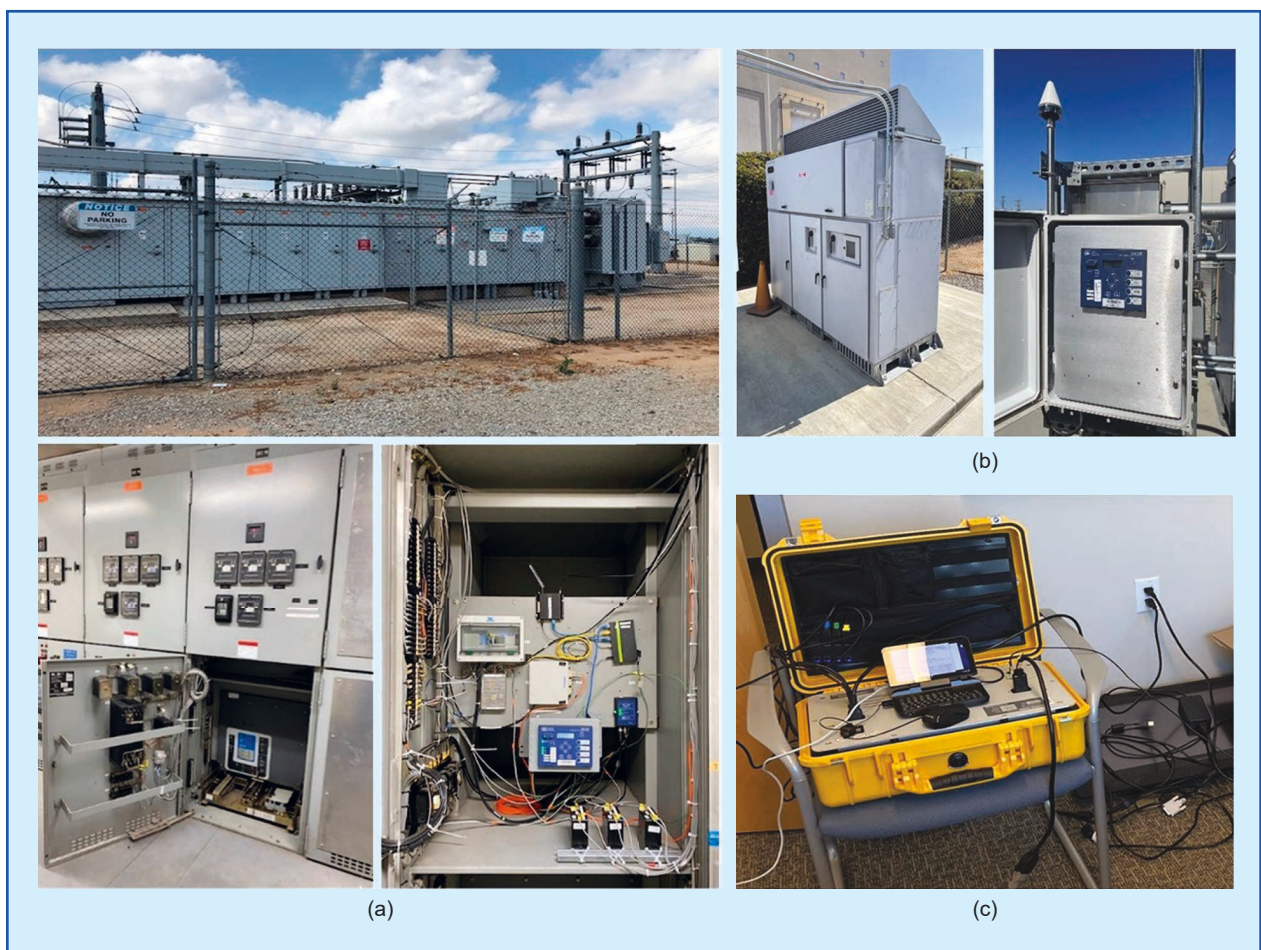
figure 2. Examples of real-world experiments in Riverside, CA, USA, to obtain synchro-waveform measurements. (a) Three-phase 12.47-kV installation at a substation. (b) Three-phase 480-V installation at a solar photovoltaic inverter. (c) Single-phase 120-V measurements at a power outlet. Photography by H. Mohsenian-Rad, P. Khaledian, H. Gomez, and Z.J. Ye.
